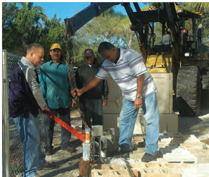
Facilities and Horticulture Team working on the South Wellhouse: Jack, Mario, Jesse, Ansel and Lee (on the loader).
